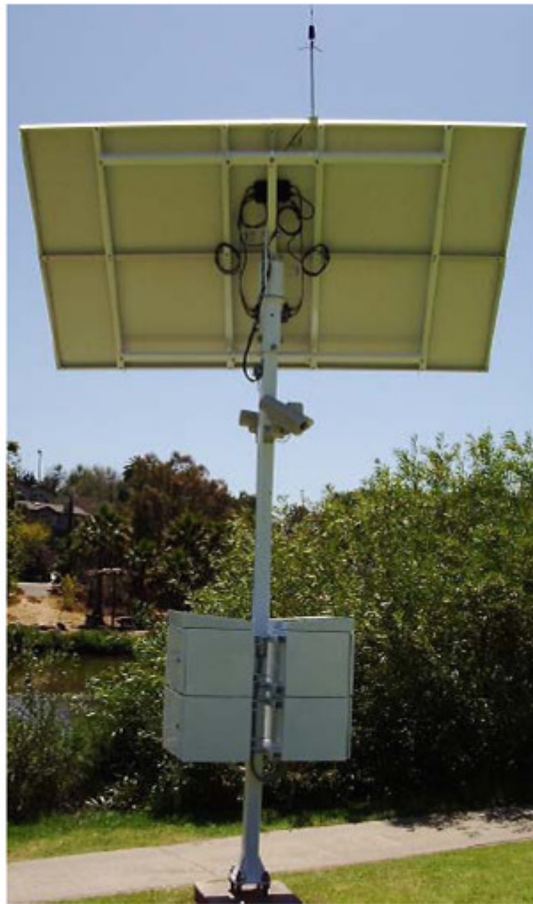
12 Foot pole with solar
