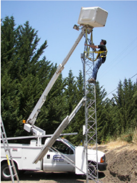
20 Foot tower with solar
