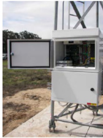
Two MOD-BOX system with Grid tie UPS
