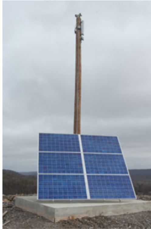
Ground Mount Solar system
